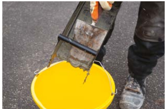
4. Remove any remaining ZeroPlus mortar from the trough before thoroughly washing that out also.
