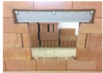
3. The lintel can then be built in using traditional mortar and again using boot cuts where possible.
